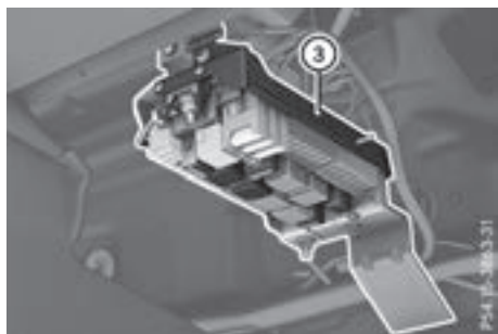
③ Fuse box
